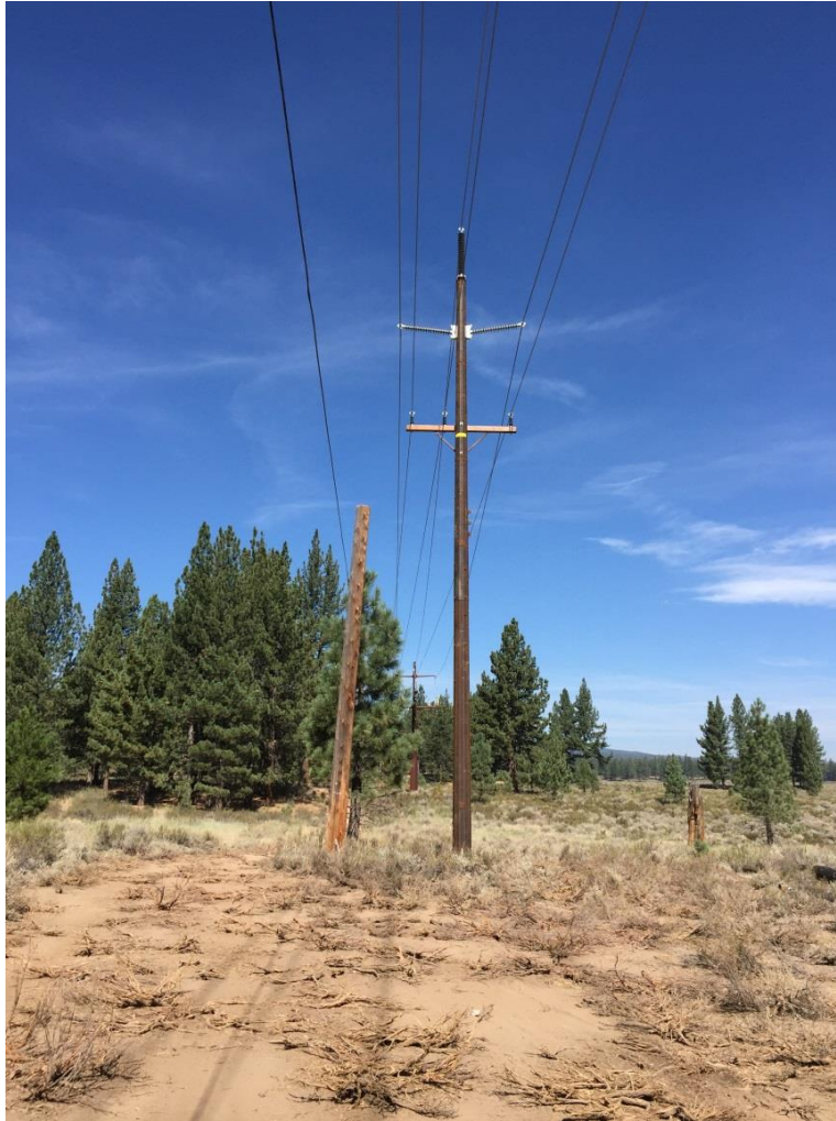
Photo 4: New weathered-steel pole installed at the northwest end Line segment 650-4. Old pole top has been and is laying in the ROW prior to removal from the project site.
