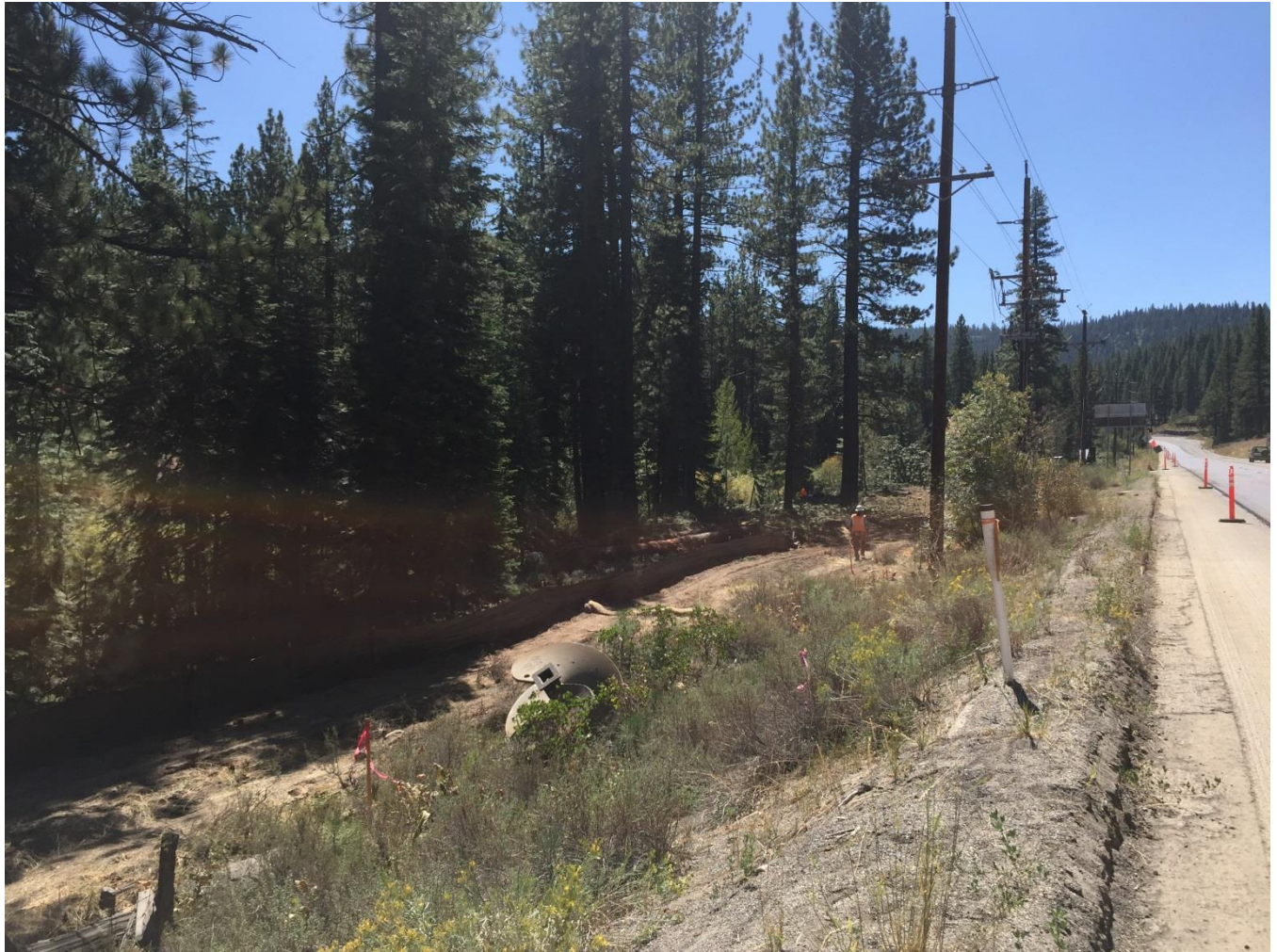
Photo 6: Tree removal activities underway between Poles #291101 and #291105. Silt fence installed along the lower edge of the ROW.
