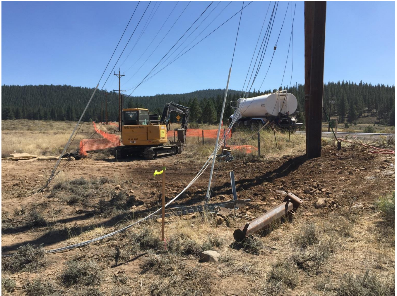
Photo 5: Construction crews setting anchors at corner Pole #291068, across SR 267 from Martis Valley. Cultural and environmental monitors present. Water truck nearby for dust control, consistent with APM-AQ-2.
